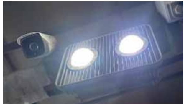
BRL's LED lighting system at Bharuch plant
