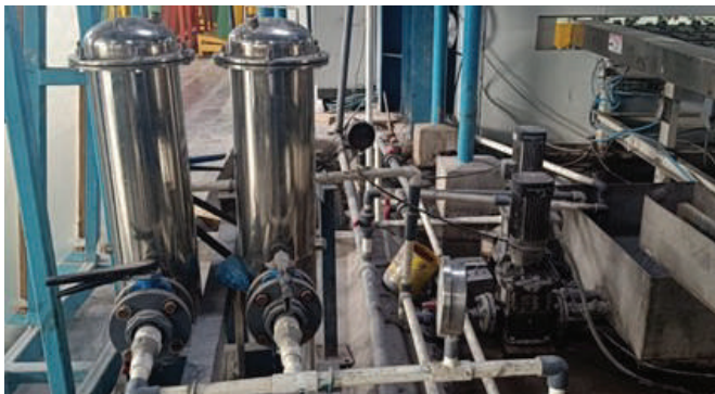
Filtration units for glass washing
